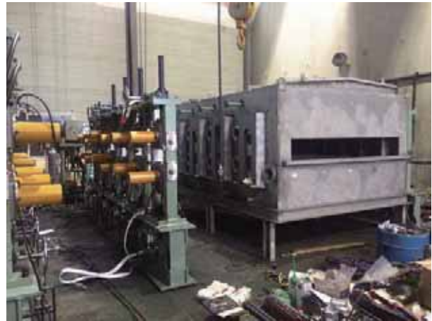
ICAL #2 BRUSH SCRUBBER TANK
